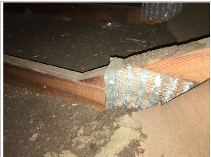
Toe Nail - Straps not meeting nail requirements
